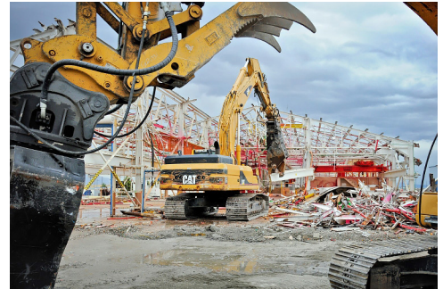
FIGURE 8: Demolition of CPP 601-602 at the Idaho site. Photo courtesy of U.S. Department of Energy.
