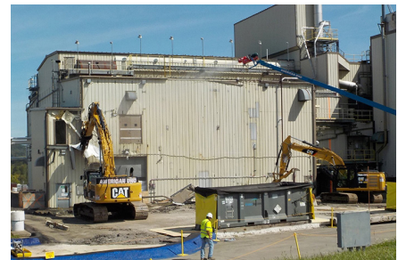
FIGURE 2: Demolition of the West Valley Vitrification Plant. Photo courtesy of U.S. Department of Energy.
