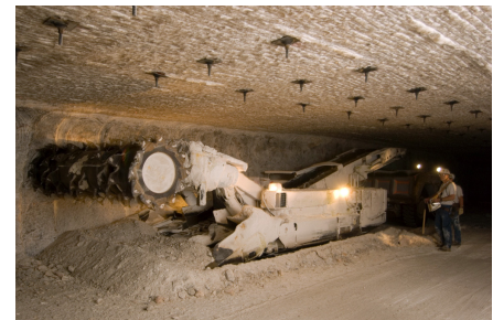
FIGURE 3: Excavation of the WIPP disposal room. Photo courtesy of U.S. Department of Energy.
