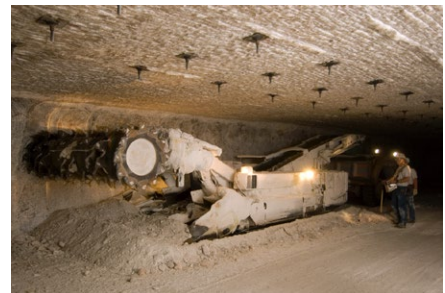
FIGURE 3: Excavation of the WIPP disposal room. Photo courtesy of U.S. Department of Energy.
